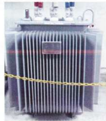
200kW/60Hz, 660V-3φ/100V-3φ, Conventional Si-Fe Transformer in TTI(1993) 1050mmH × 700mmW × 1100mmL
